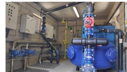
WATER RECLAMATION PLANT
